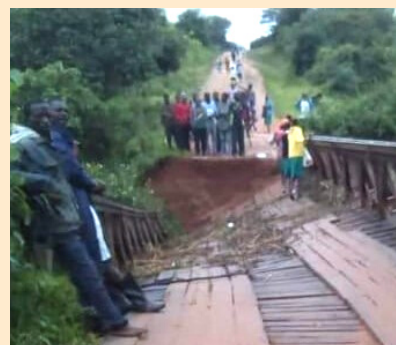
Mzambazi bridge after heavy rains
